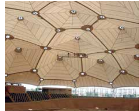
Velodrome - Abuja, Nigeria Engineer: form TL Fabricator: Canobbio Labor Blum: Production, third-party and installation monitoring, quality control
