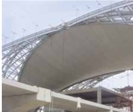
New Bangkok International Airport - Bangkok, Thailand Engineer: Werner Sobek Stuttgart GmbH & Co. KG Fabricator: Hightex GmbH Labor Blum: Incoming goods control, quality assurance
